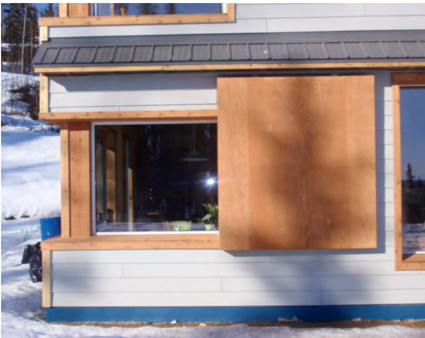
Figure 6. A close-up view of the shutter system on the Chlupp residence. This is only one of the largest of several shutter types that Chlupp used in his home. This one slides on a garage door slide system (a sort of pocket-door arrangement) so that the shutter is always exposed on the house wall outside. In other parts of the home (not shown) shutters are designed for use on the inside of the windows and slide into the wall when not in use and are out of sight.
