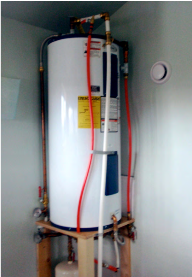
Figure 11. The water tank/heater is located on the third floor to allow for thermosiphoning of heated water from the masonry stove.
