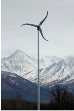
Installed turbine at Sherrod Elementary in Palmer, AK
