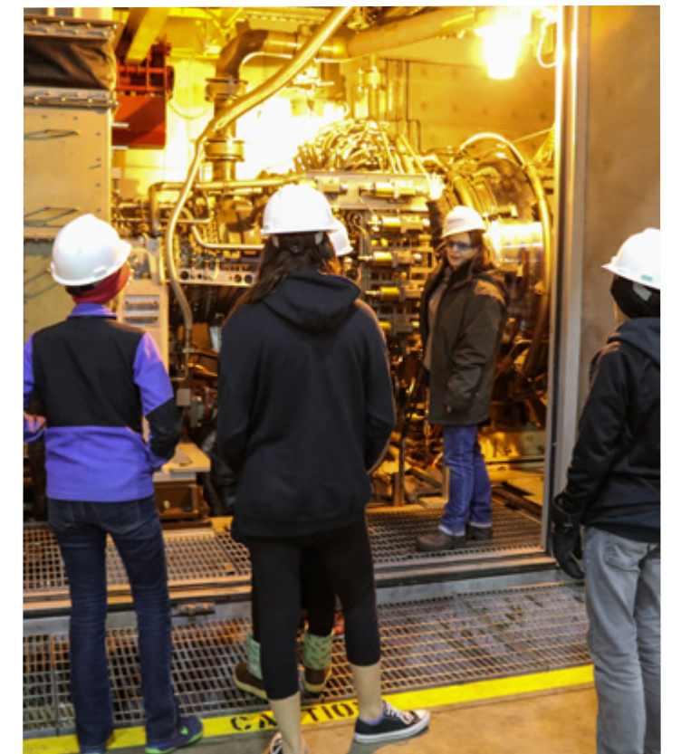
Power Pledge Challenge winner's tour of the Matanuska Electric Association powerplant. Photo courtesy of REAP.
