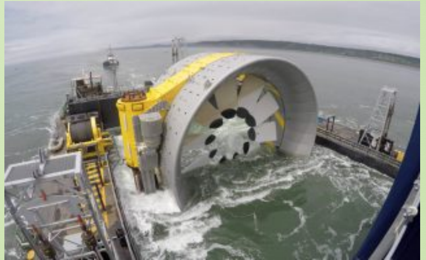
A 2MW OpenHydro tidal turbine installed in Canada in July 2018 (Photo: Cape Sharp Tidal)
