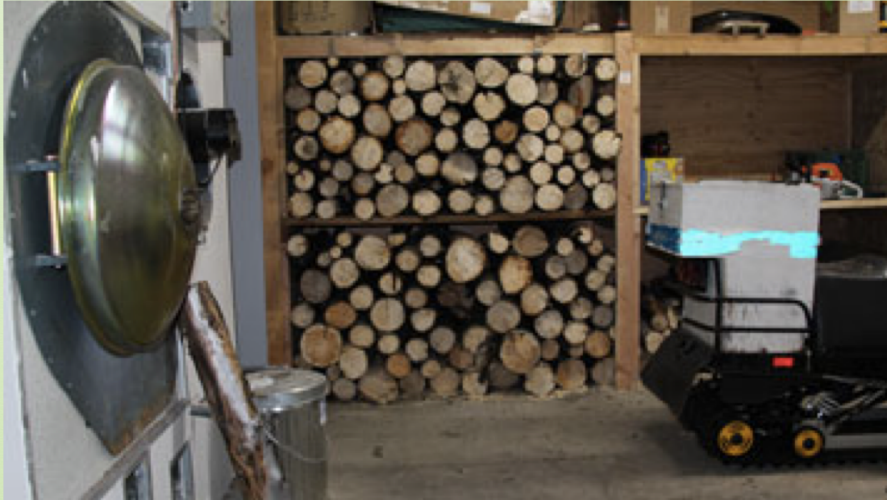
The biomass system and cordwood storage in Tanana, Alaska. Photo courtesy of Tanana Fire Department.
