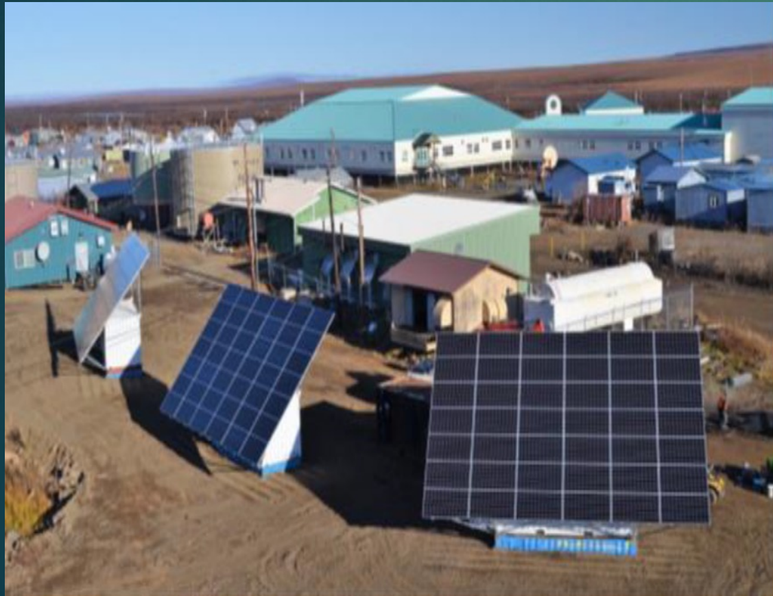
Buckland Solar arrays, Courtesy NANA
