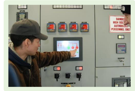
Monitoring generator performance.
