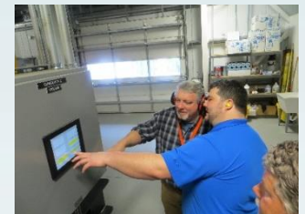
Looking at generator performance. (Photo credit: AEA)
