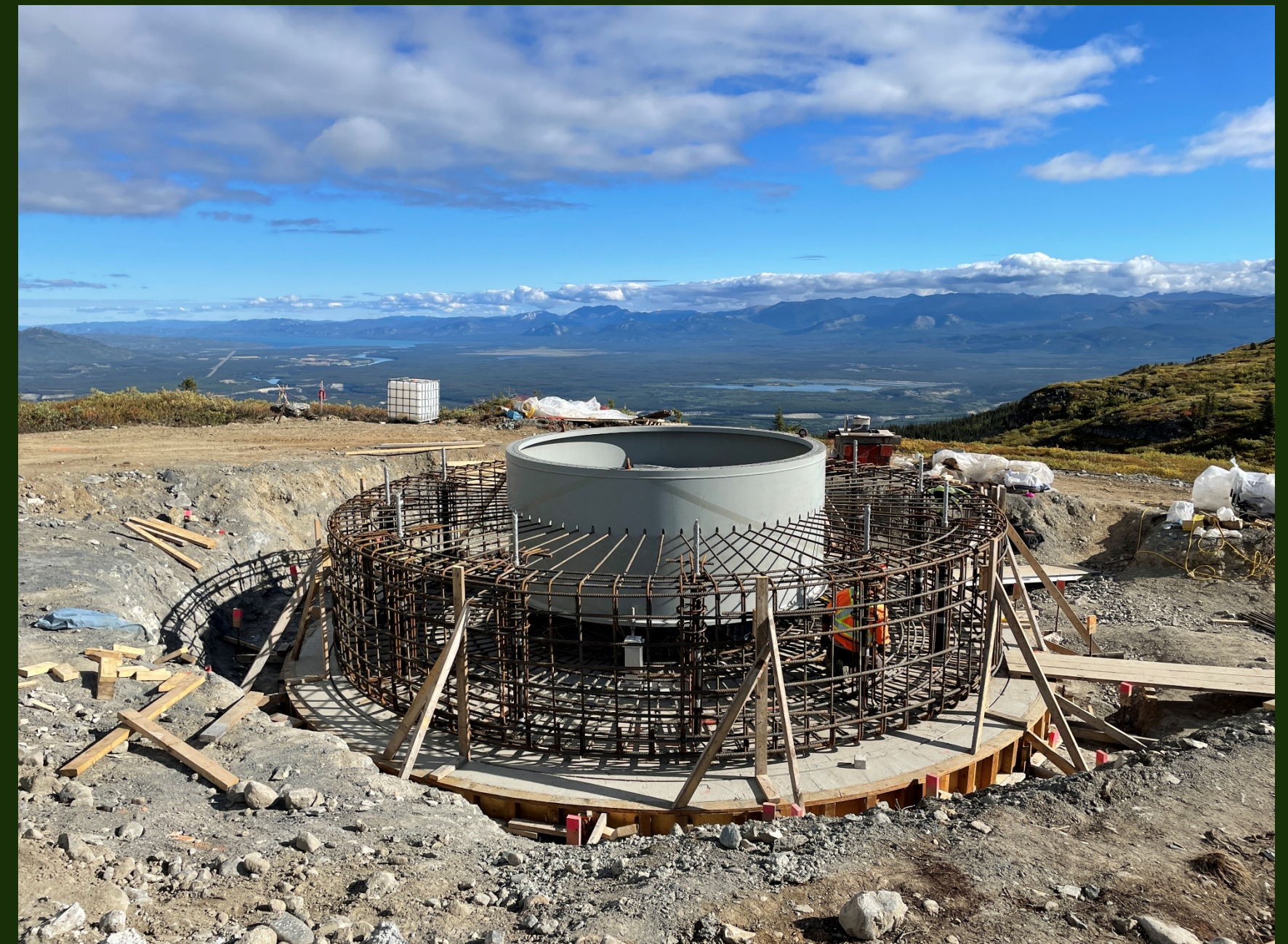
Construction that can be done in cold climate and span over multiple years
