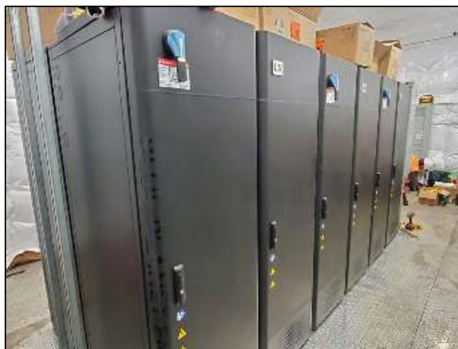
Figure 30. Batteries for Shungnak, Prior to Installation (Photo Courtesy of Ingemar Mathiasson)
