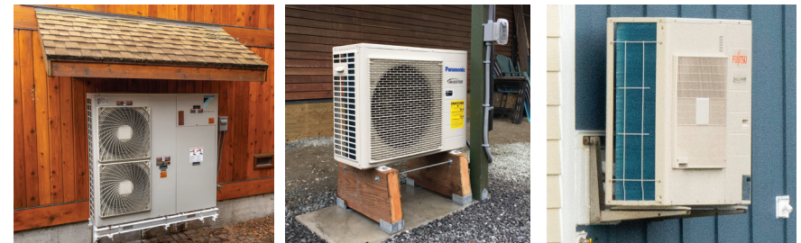
Examples of snow-protected outdoor units—under roof, on elevated blocks, and wall-hung units
