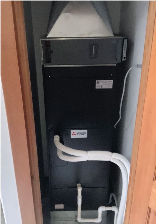
Just like a furnace, this indoor air handler blows warm air throughout the home through ducts. The refrigerant lines (paired white lines in this photo) connect the air handler to the outdoor unit.
