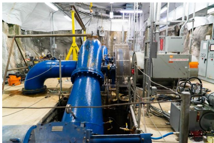
Iliamna-Newhalen Electric Cooperative's Tazimina hydroelectric plant is one of many renewable energy generation projects in the state that has received support from the Renewable Energy Fund. Photo: Emma Hamilton/REAP
