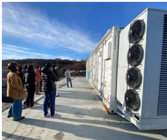
A student group visits a battery energy storage system in Nome. Photo: Jenny Starrs/REAP
